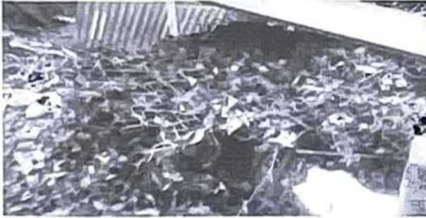
Cyclone Wire Picture # 54
